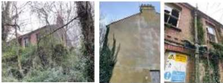
Existing 'Lime Kiln Cottages' – Broken windows and overgrown
